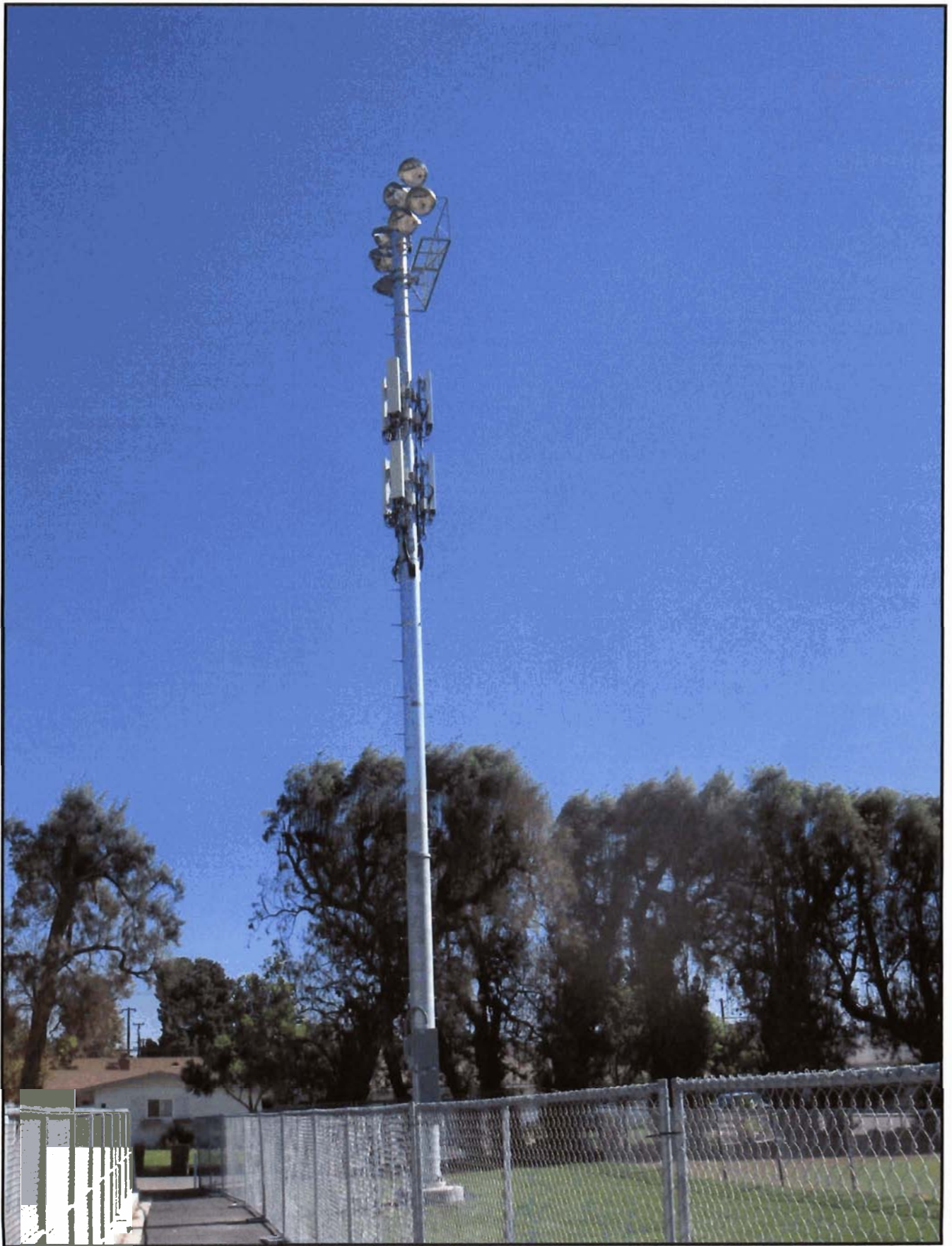
Pleasant Valley Park in Camarillo (Underground Vault)
